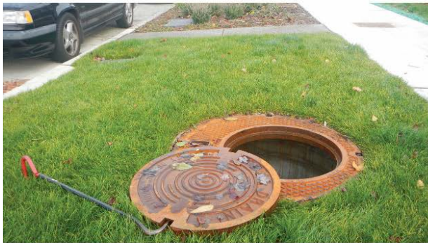
UMH has dual access opening (3’ and 2’ dia.) for meeting routine maintenance requirements and opening with MH lift rod. Level area around MH allows space for crews to remove lid.
