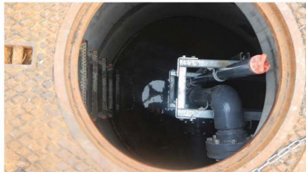
UIC Maintenance Hole
