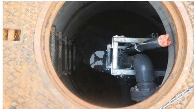
UIC Maintenance Hole
