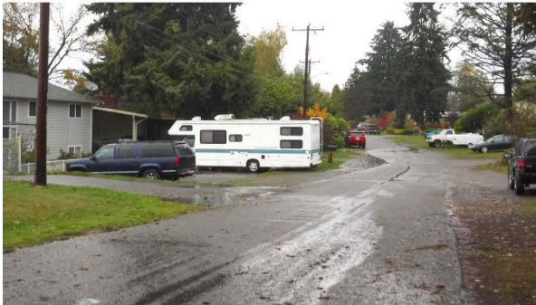
Narrow existing pavement width and localized flooding
